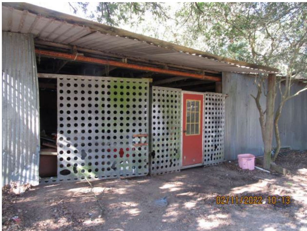
Code Enforcement inspection photograph (February 16, 2022).
