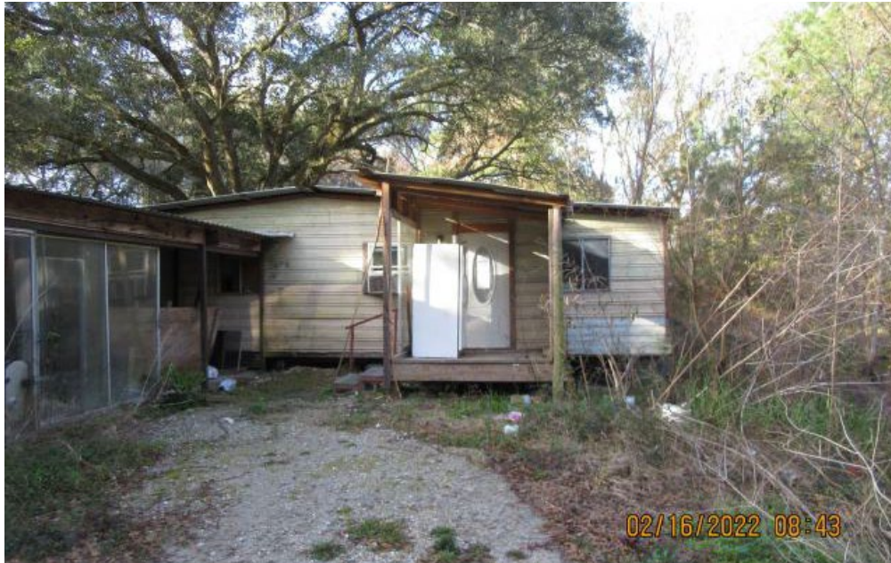
Code Enforcement inspection photograph (February 16, 2022).
