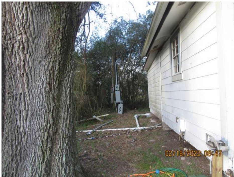
Code Enforcement inspection photograph (February 16, 2022).
