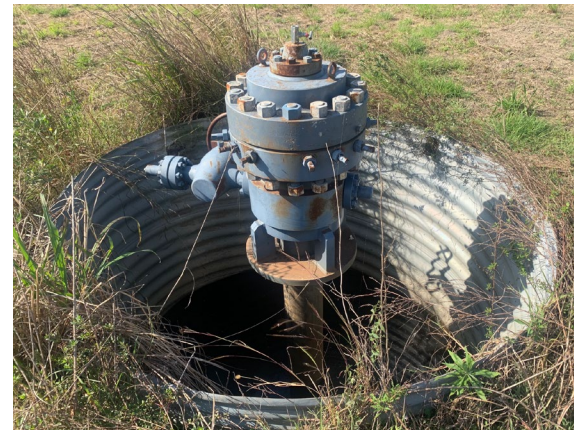
Existing Scout #1RE Wellhead
